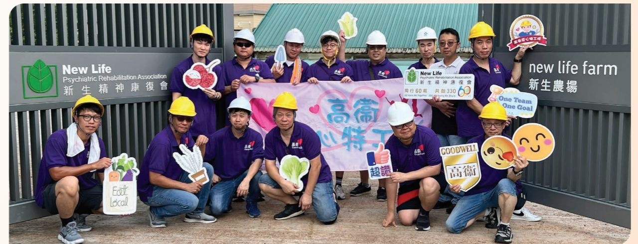
On 6 September 2025, volunteers of Goodwell's Technical Management Committee made good use of their profession in technical field to conduct basic repairs in the indoor activity rooms and painting work of the outdoor wire fences for New Life Farm, Hong Kong's first eco-tourism farm run under a social enterprise model.
