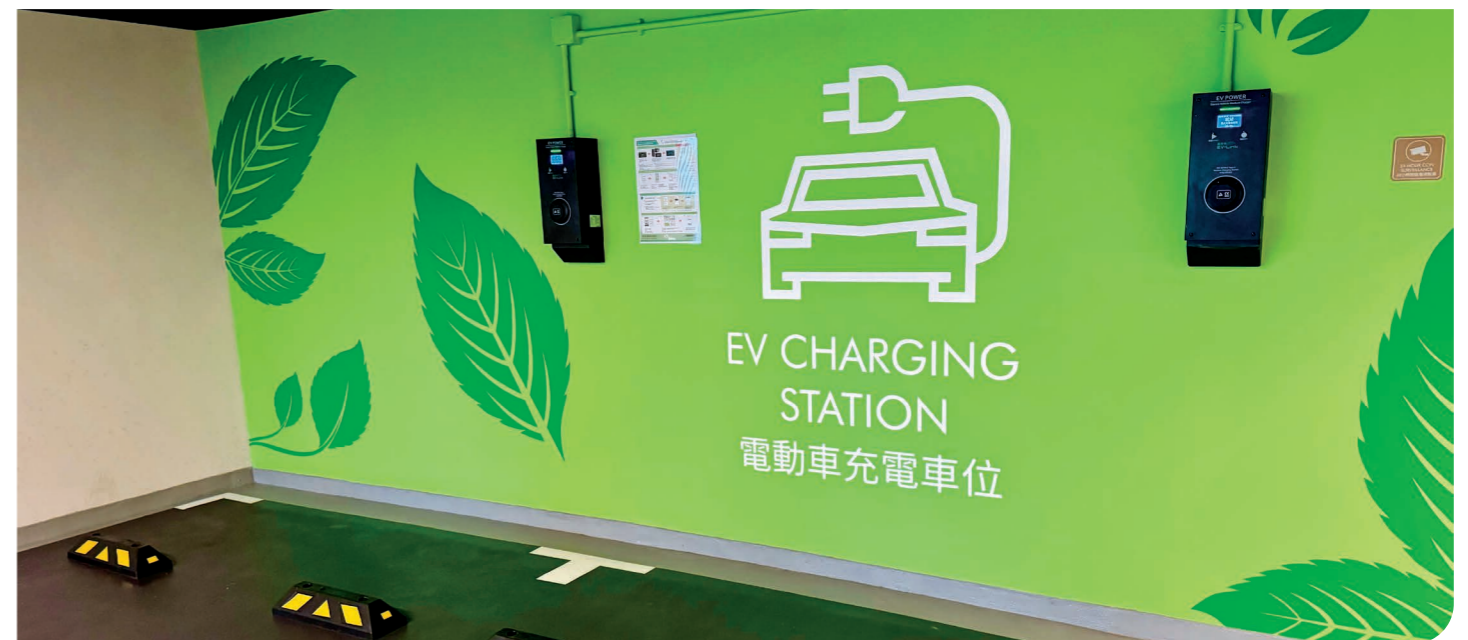
EV chargers are installed in car parks of Cheung Kong Center II to advance the sustainability initiatives.
