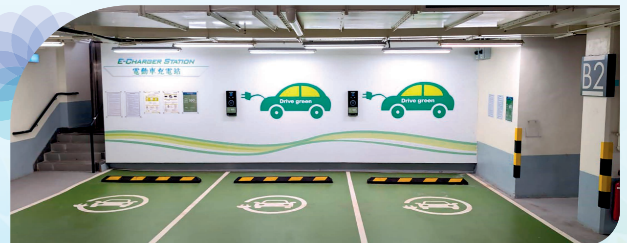
EV chargers are installed in car parks of Cheung Kong Center to advance the sustainability initiatives.
