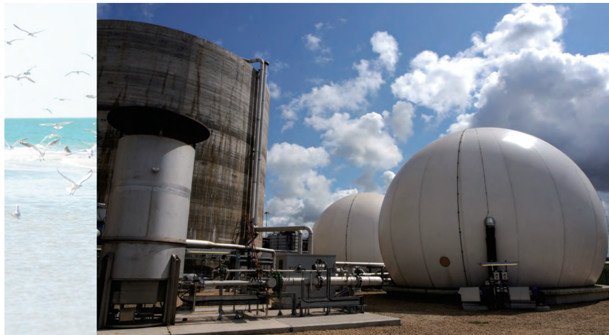
Northumbrian Water's Sludge Treatment Centre at Howdon.
